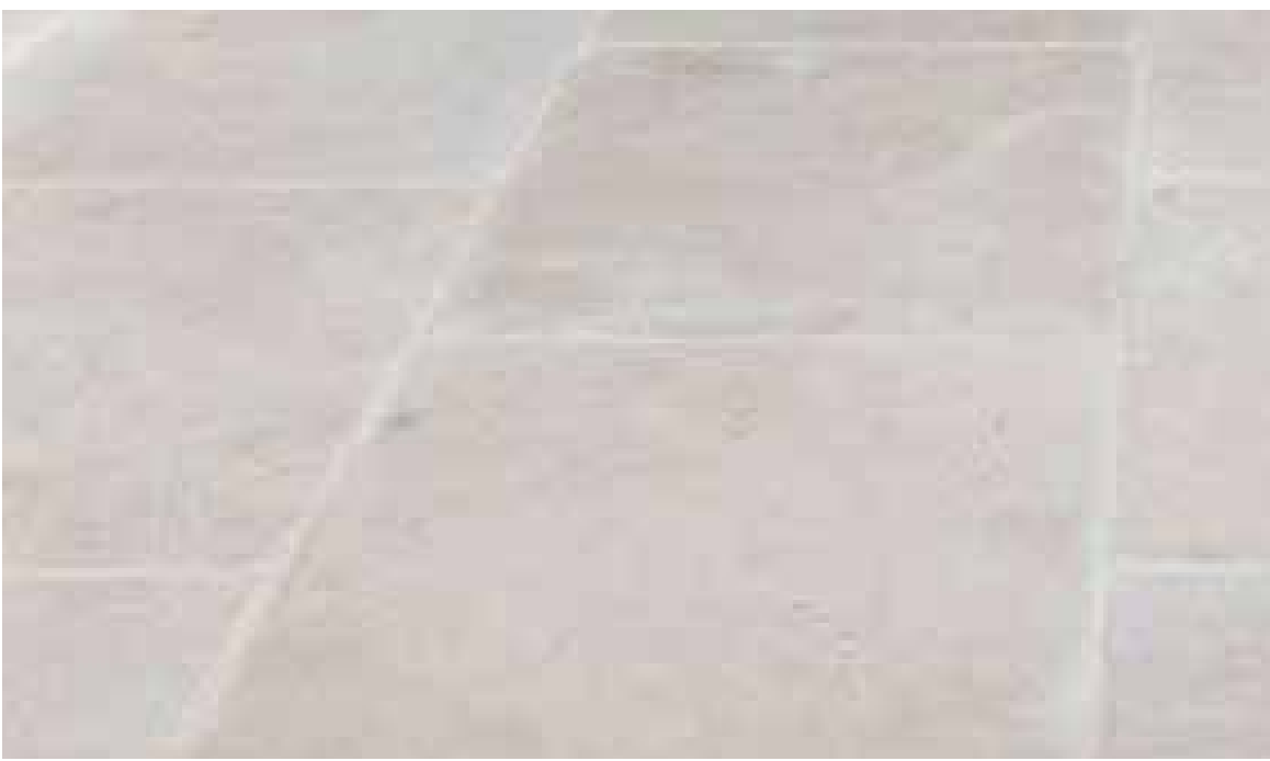
Private terrace tile paving
